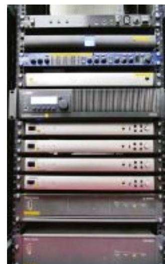
Four FreeSpace IZA 2120-HZ models and a single PowerMatch PM-4250 amplifier power the Bose speakers
